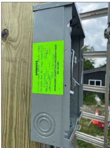
Meter socket inspection sticker.
