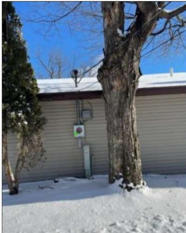
Approved overhead service, meter set only.
