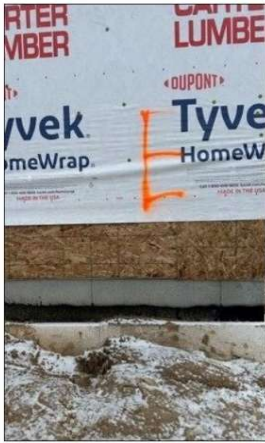
Meter location marked.
